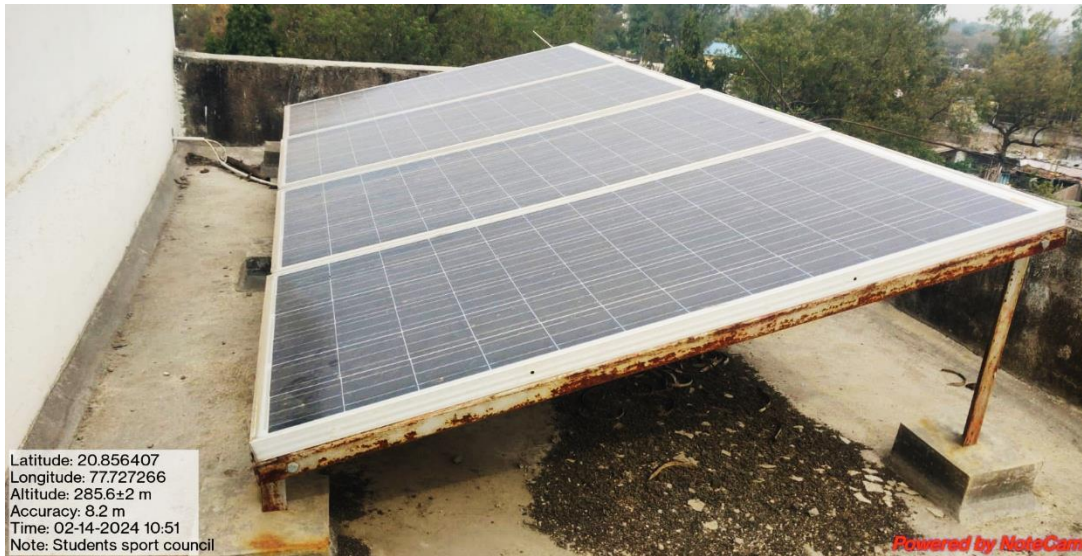
Solar panels (1.1 KV)
