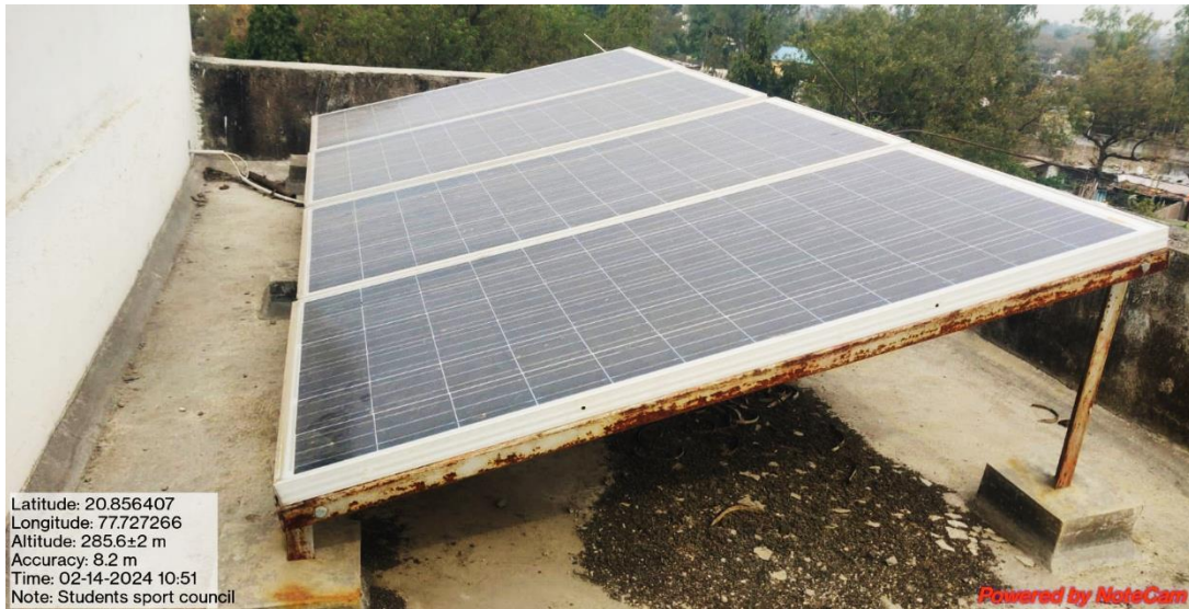
Solar panels (1.1 KV)
