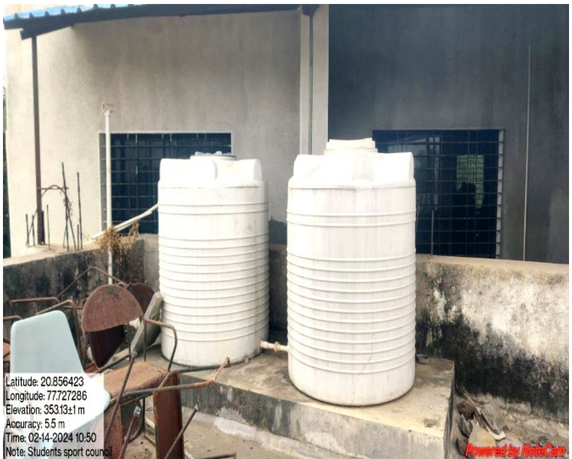
Water Storage System
